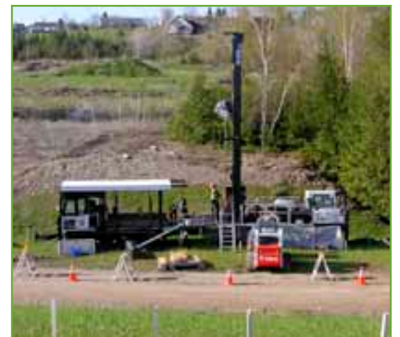
With more than 500 bores, wells, probes, and screens installed, and more than 7,000 water readings taken, East Park and Bay Harbor are perhaps the most studied pieces of property in northern Michigan.
